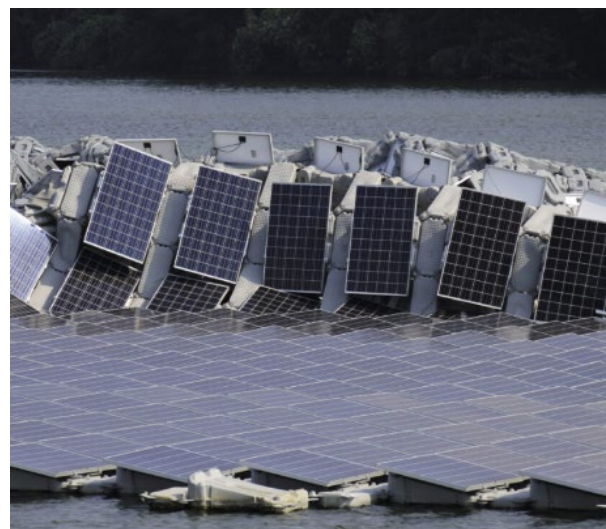
Fig 1: Failure of a FPV system ( https://solaredition.com/destruction-of-floating-pv-plant-by-typhoon-at-yamakura-dam-wind-resistance-in-spotlight )
